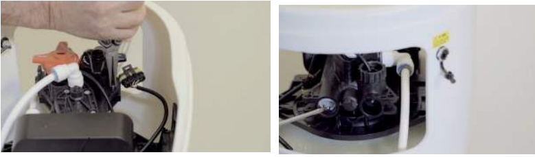
Water inlet filter replacement
